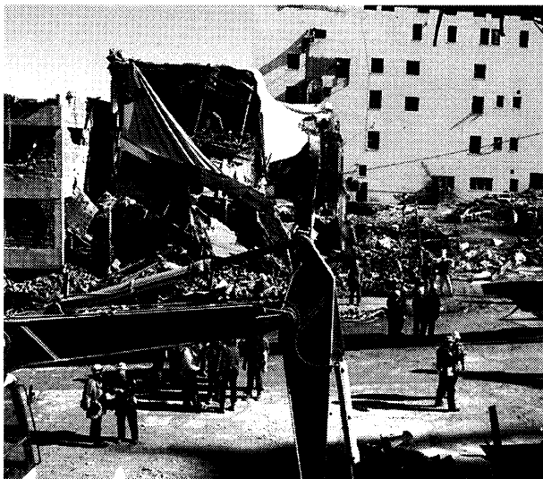
A trackhoe removes debris while USAR and other crews observe from the street. The Water Resources Board and the collapsed Athenian Building, along with the crushed and burned cars in the parking lot are seen. The Journal Record Building rests in the background.
